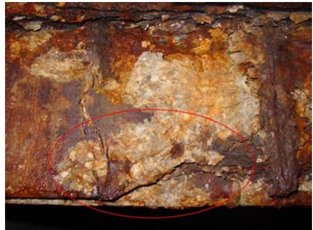
Figure 6. Corrosion due to chemical compounds
