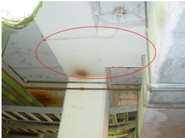
Figure 5. Absence of beam to column connection
